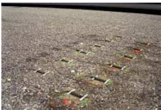
Horizontal strain sensors on GB base.
